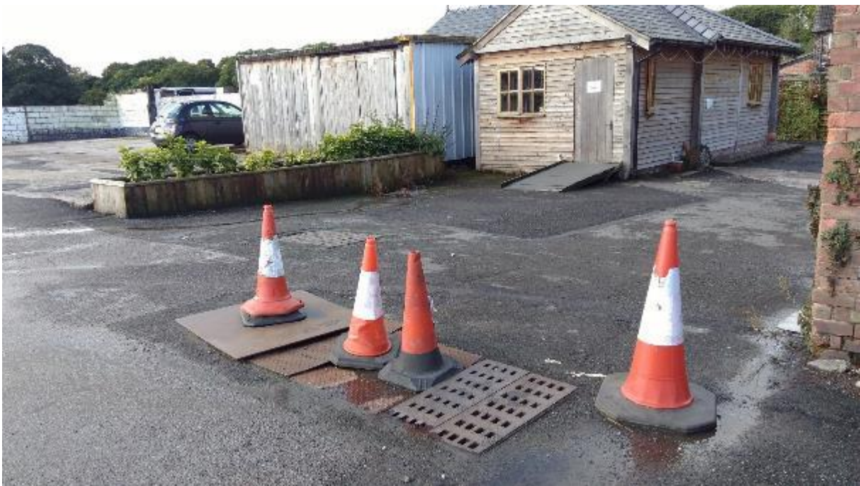
Photograph 6 – Covers for surface water drains, understood to feed to Dood's Brook to the south-west
