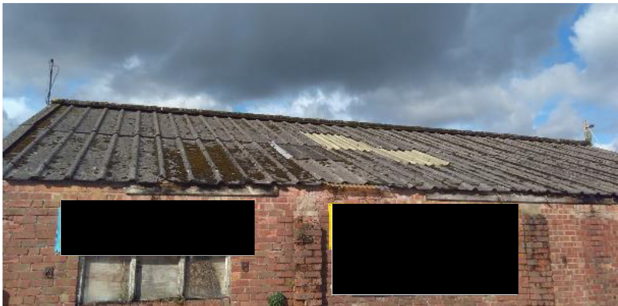
Photograph 2 – Suspected asbestos roof panels on barn building
