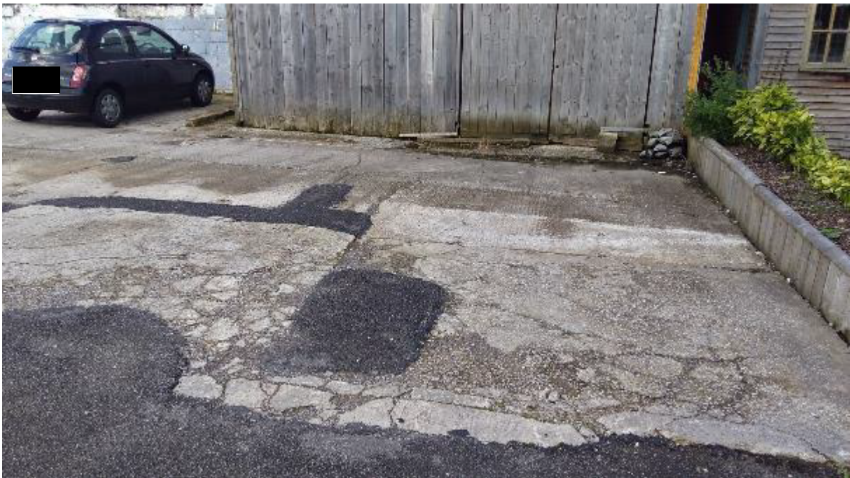
Photograph 10 – Hardstanding in poor repair across Site
