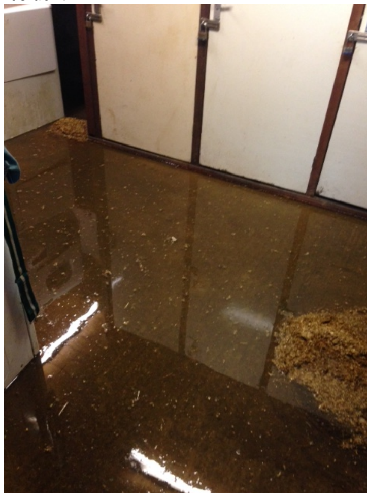
Figure 4: Image of flooding on 26 December 2015 to stable block provided by resident.
