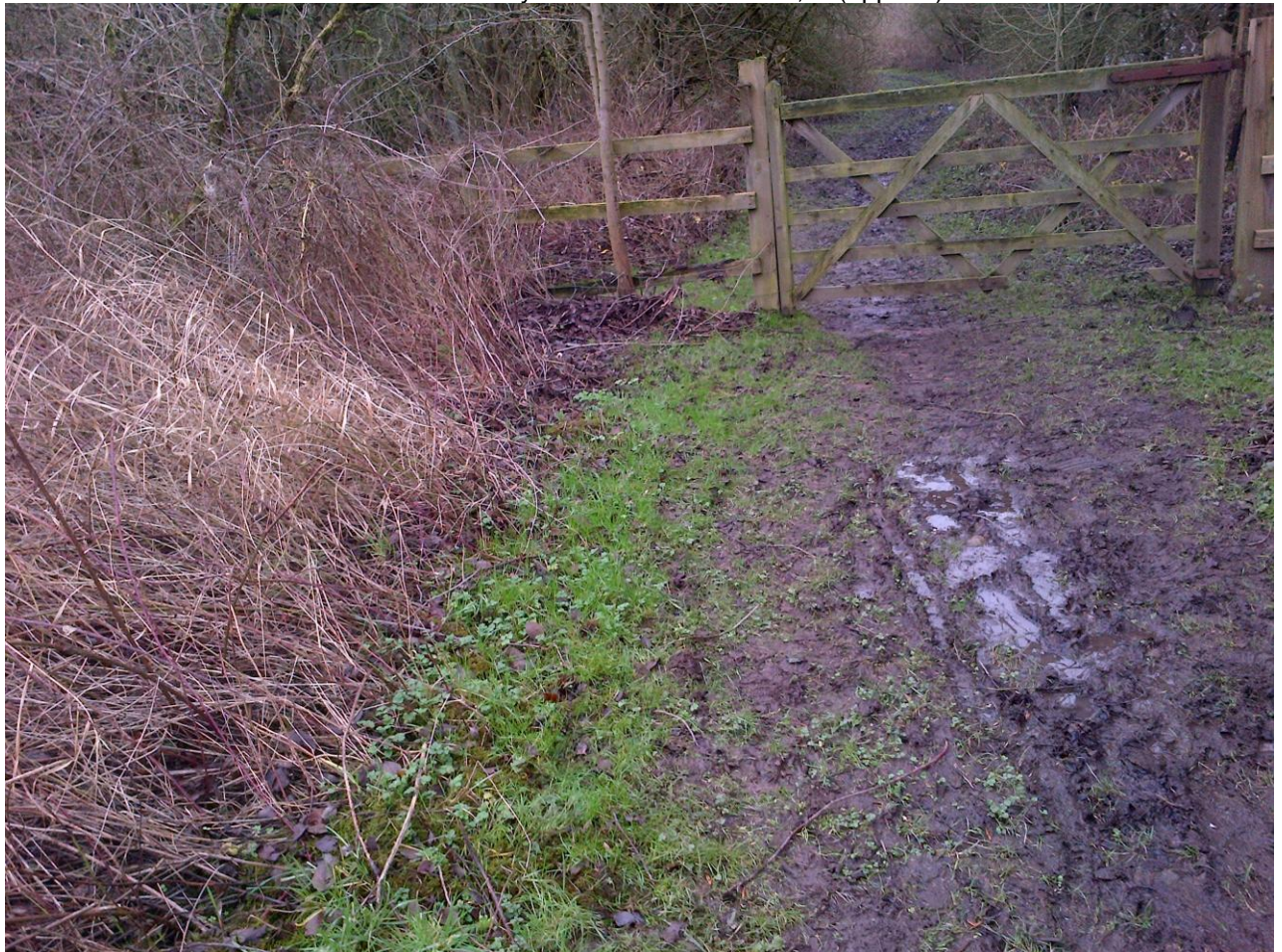
Photo 4) Overtopping embankment low spot. From SJ6607088077, West.
