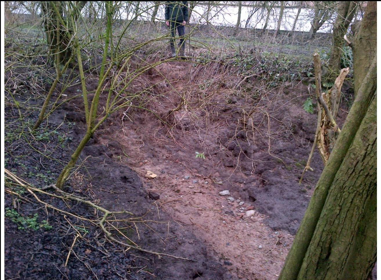
Photo 5) More significant overtopping embankment low spot. From SJ6601388046, North.
