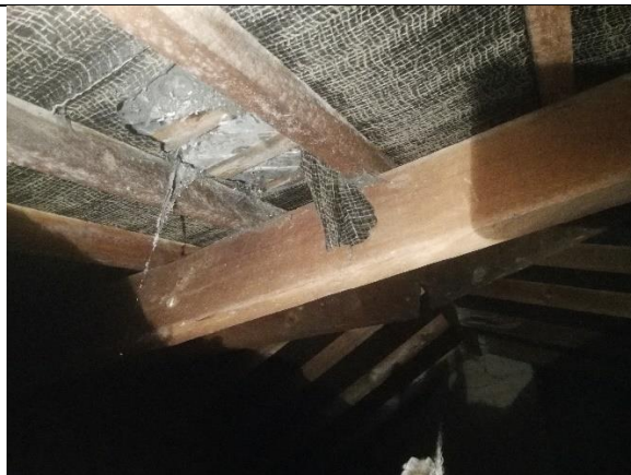
Photograph 28: Densely cobwebbed tears in the plastic lining near the access hatch within the loft of 460 Poplars Avenue.
