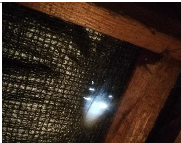
Photograph 20: Densely cobwebbed hole near roof apex (344 Poplars Avenue)
