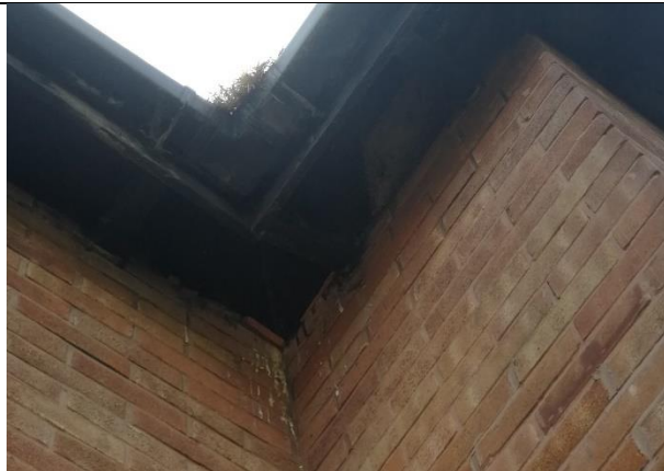
Photograph 2: Nest in guttering seen from below with liming evident (344 Poplars Ave.)
