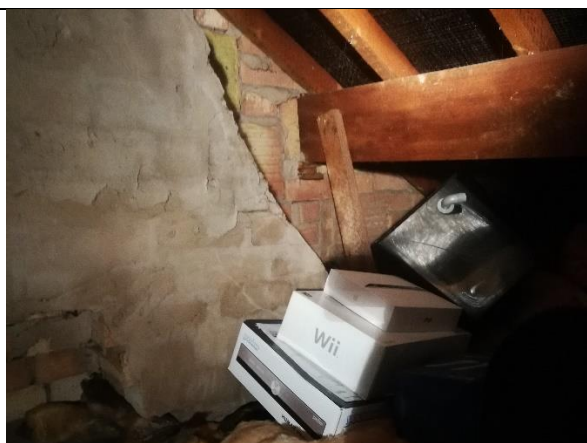
Photograph 24: General character of 458 Poplars Avenue, showing partition wall and chimney breast shared with 456 Poplars Avenue.
