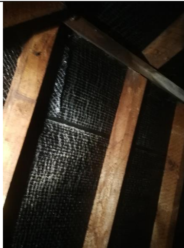
Photograph 26: Overlap gap between plastic lining layers within the loft of 458 Poplars Avenue
