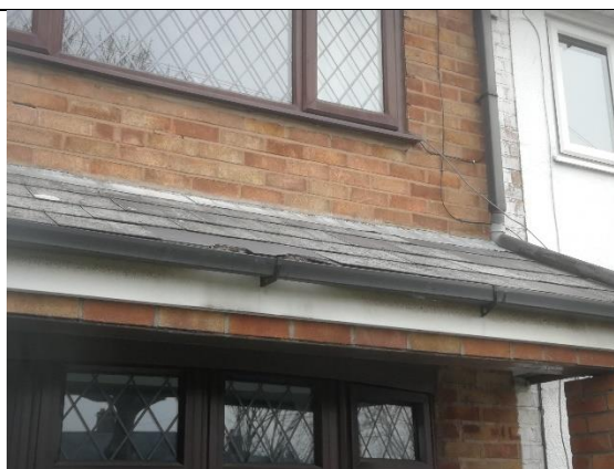
Photograph 10: Broken and lifted slates on porch roof (458 Poplars Avenue)
