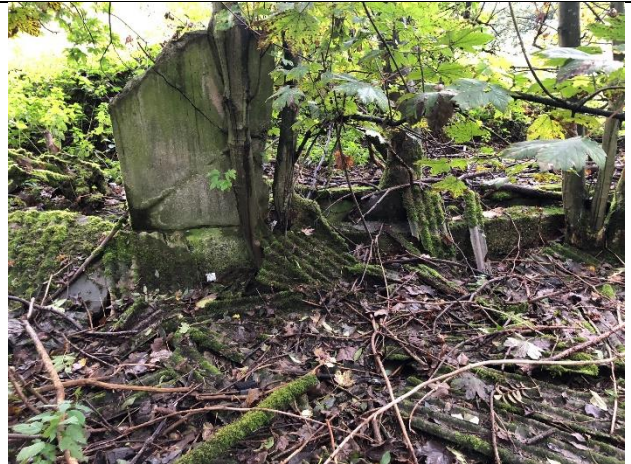
Photograph 51: Rubble remaining from a demolished farm outbuilding, inclusive of asbestos roofing materials; Compartment G
