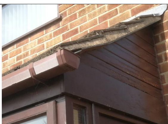
Photograph 4: Gap present at driveway side porch eave (344 Poplars Ave.)
