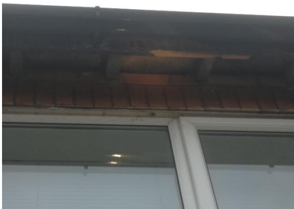
Photograph 15: Gap where wall meets eaves at rear of house (462 Poplars Avenue)
