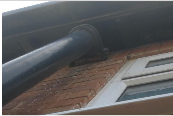
Photograph 18: Liming present indicating a gap not visible at ground level between the top of the wall and the eaves (464 Poplars Avenue).
