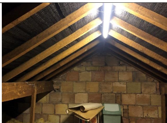
Photograph 22: Partition wall shared with 350 Poplars Avenue with gaps around rafters
