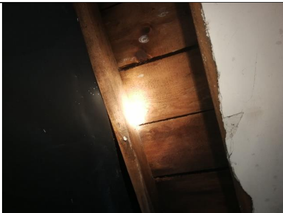
Photograph 50: Roof of outbuilding associated with 462 Poplars Avenue, showing liner and signs of dampness
