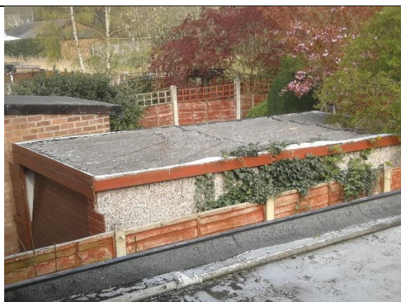
Photograph 44: Garage associated with 460 Poplars Avenue (as seen from the upstairs window of 458 Poplars Avenue)
