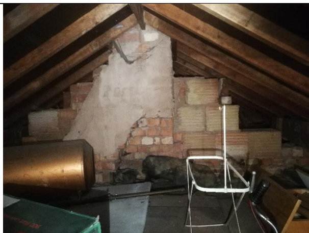
Photograph 19: Partition wall with large gaps between wall and roof (344 Poplars Avenue)
