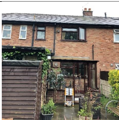
Photograph 7: Small porch of brick and glass with wood framing and a plastic sheet roof (348 Poplars Avenue)
