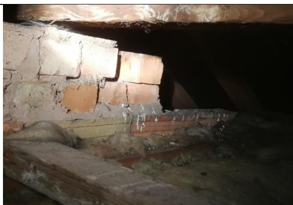
Photograph 21: Liming at partition wall indicating a hidden loft access used by birds (344 Poplars Avenue)
