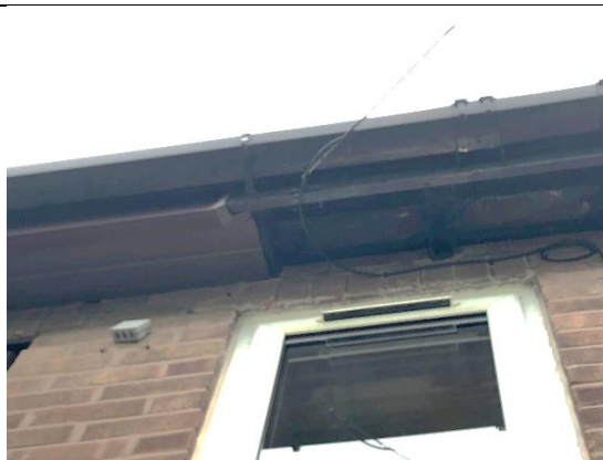
Photograph 8: Uncapped boxed soffit ending at adjacent property (348 Poplars Avenue)
