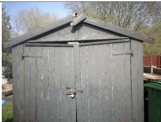
Photograph 35: Wood panelled doors with large gap present (344 Poplars Avenue)
