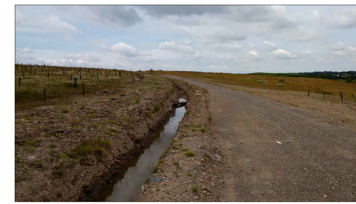
PHOTOGRAPH 9 : STANDING WATER IN DITCH WITH INSUFFICIENT GRADIENT
