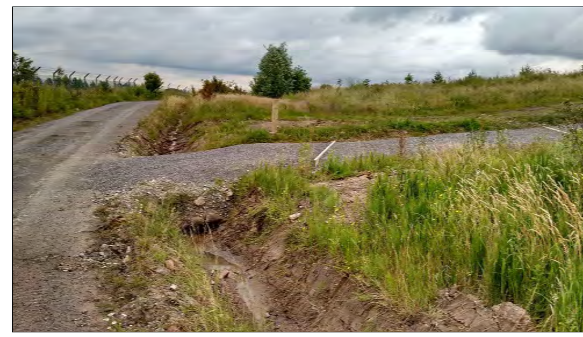
PHOTOGRAPH 6 : DRAIN CONFLUENCE PRONE TO SURCHARGING
