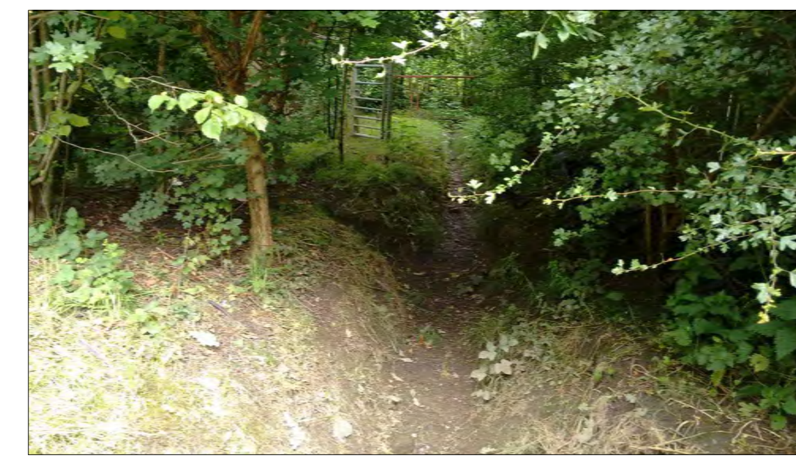
PHOTOGRAPH 11 : DITCHES AT COMPOUND PRONE TO SURCHARGING
