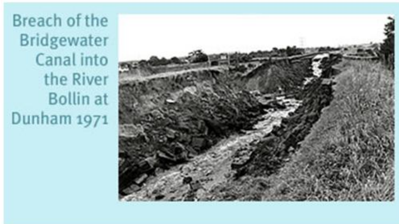
Figure 5-1: Bridgewater Canal Breach at Dunham
