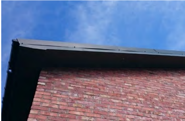
Photograph 1: Gaps under external roof cladding
