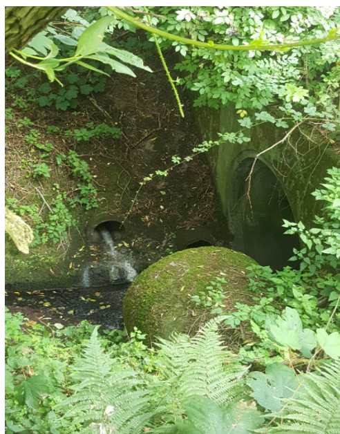
Photograph showing incoming connections to Bradley Brook
