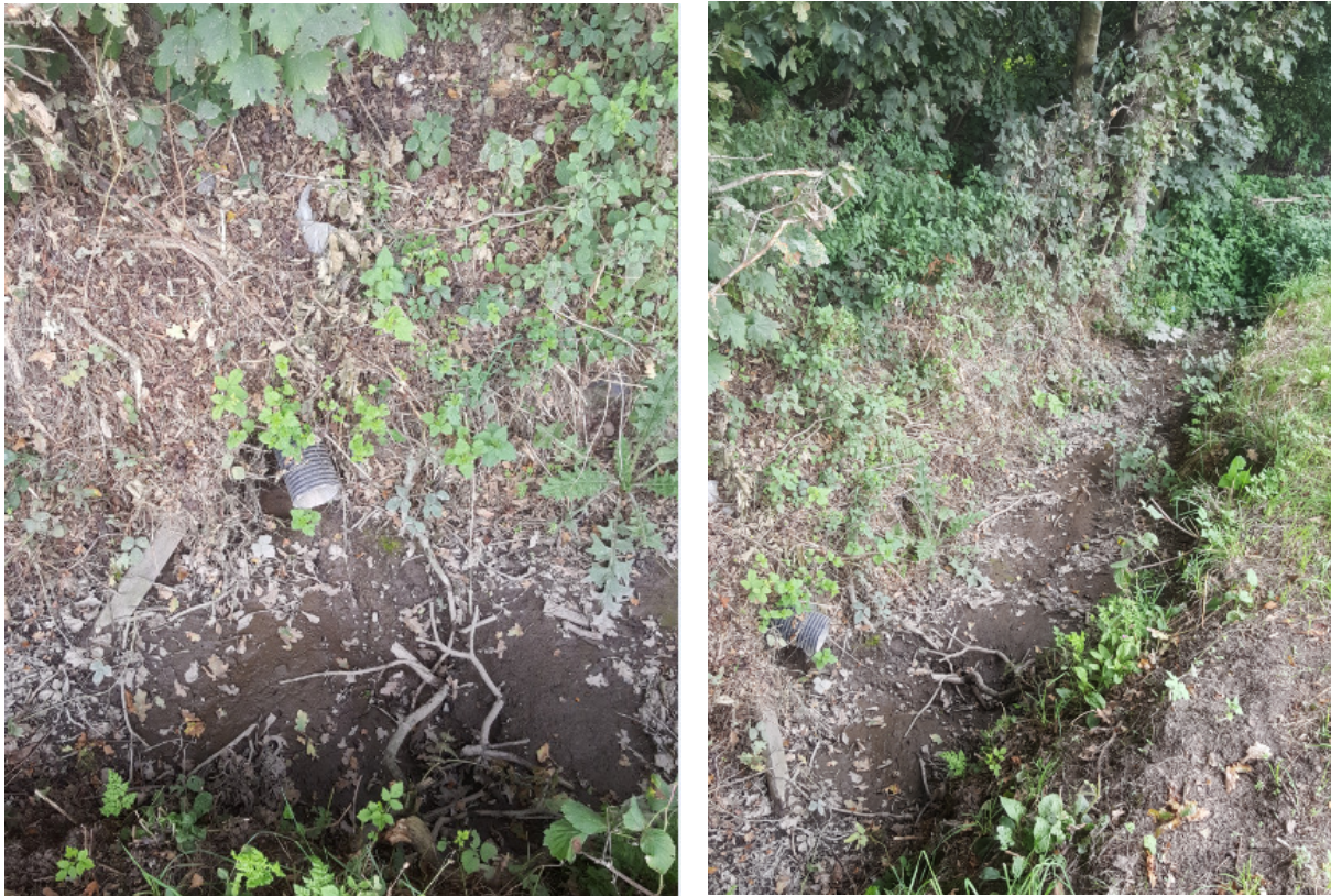
Photographs showing incoming connection to ditch (L) and ditch appearing to fall towards the northern boundary (R) but no culvert/outlet could be identified
