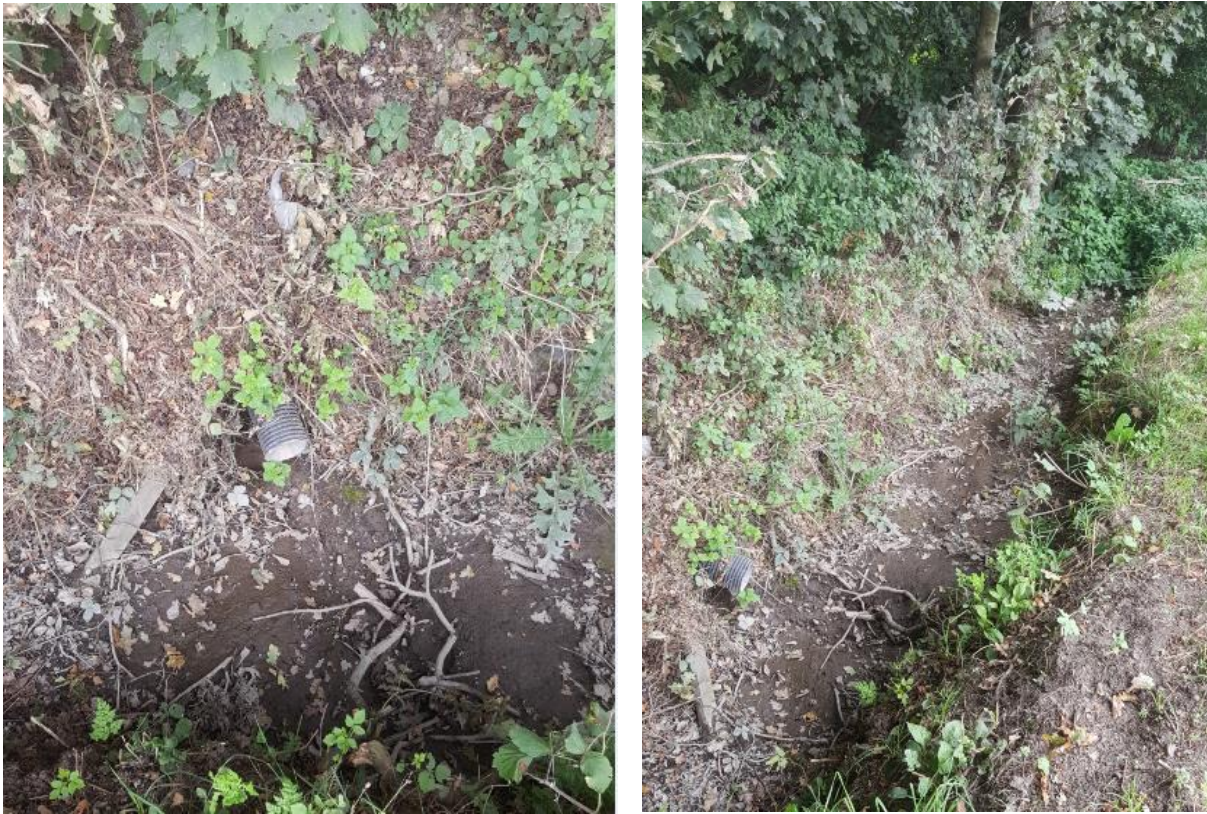
Photographs showing incoming connection to ditch (L) and ditch appearing to fall towards the northern boundary (R) but no culvert/outlet could be identified
