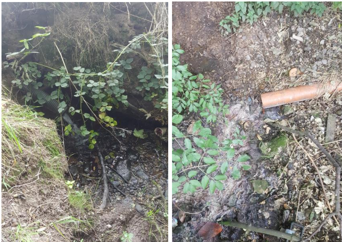
Photograph showing surface water flow to the ditch (L) and additional connection from adjacent property appears to discharge waste to head of the ditch (R)
