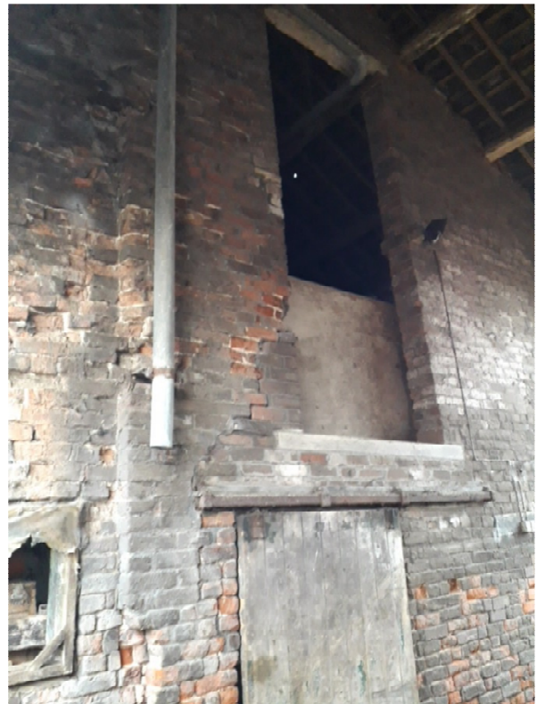
Figure 4: Cracking adjacent to existing openings
