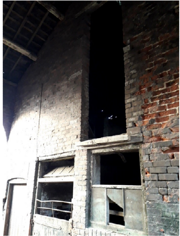
Figure 2: Extensive loss of masonry face to entrance
