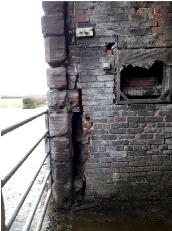
Figure 2: Vertical cracking and separation to rear of entry arch
