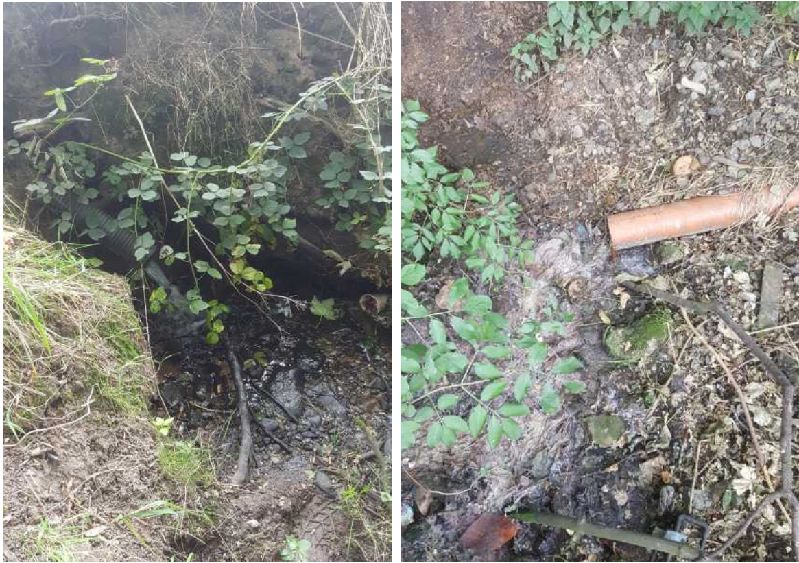
Photograph showing surface water flow to the ditch (L) and additional connection from adjacent property appears to discharge waste to head of the ditch (R)
