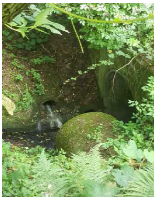
Photograph showing incoming connections to Bradley Brook
