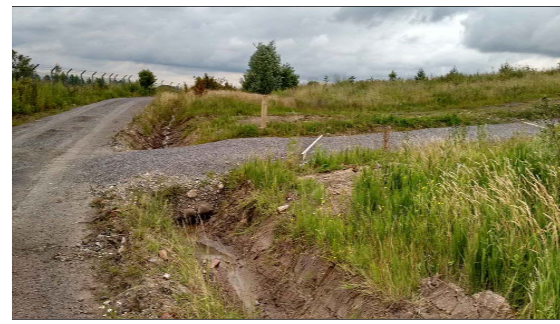
PHOTOGRAPH 6 : DRAIN CONFLUENCE PRONE TO SURCHARGING
