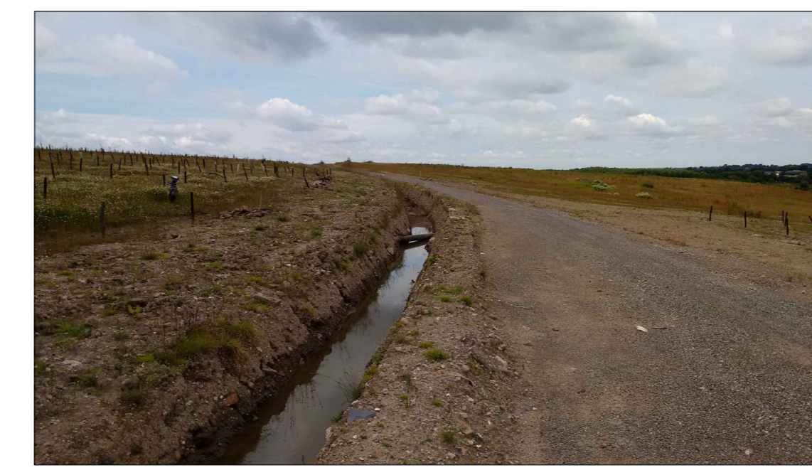
PHOTOGRAPH 9 : STANDING WATER IN DITCH WITH INSUFFICIENT GRADIENT
