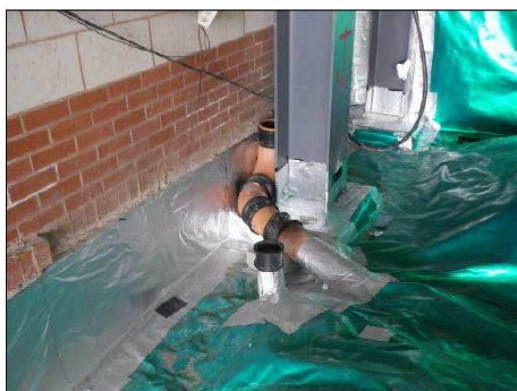
Seal pipes at 1J
