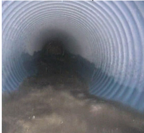
Figure 17: Extract from CCTV Survey Upon Completion of Works Showing Repairs Section of Pipe
